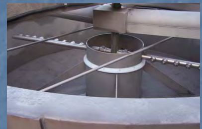
Spray Nozzles Inside Strainer
